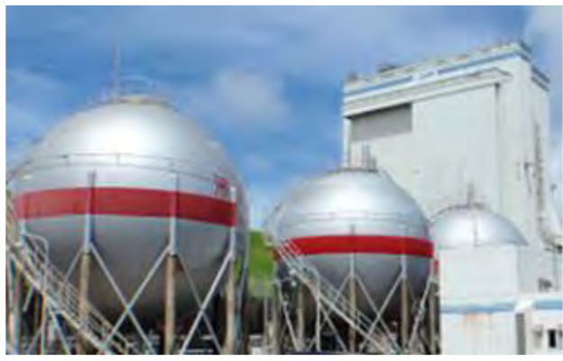
Largest liquefied hydrogen tanks in Japan (Tanegashima Rocket Base)
