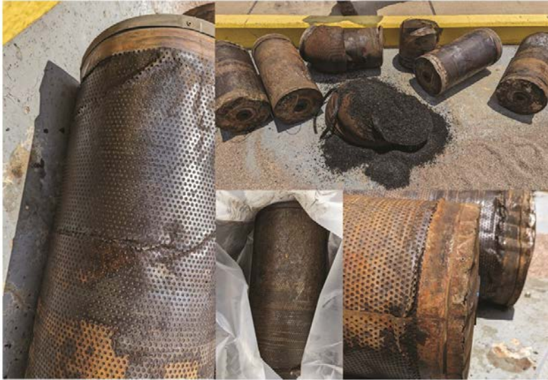
Carbon canisters removed/replaced after shutdown with \sim 1,760 hours in service. (Second set)
